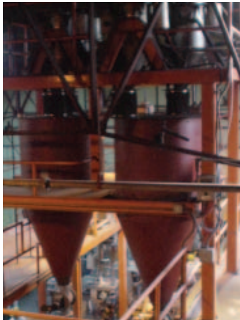
These feed hoppers deliver the blended coffee to the packaging machines. Each has two vacuum receivers that work in tandem to fill the hoppers when a level switch gives the signal. Throughput is 500 kilograms per hour.
