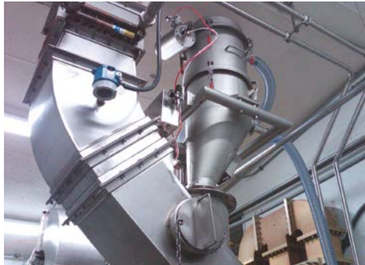
Two of the pneumatic conveyors at Nutriom are tied to a mixer, with one conveyor breaking up egg powder and putting it into the mixer and the other transferring it out. Photo: Vac-U-Max
